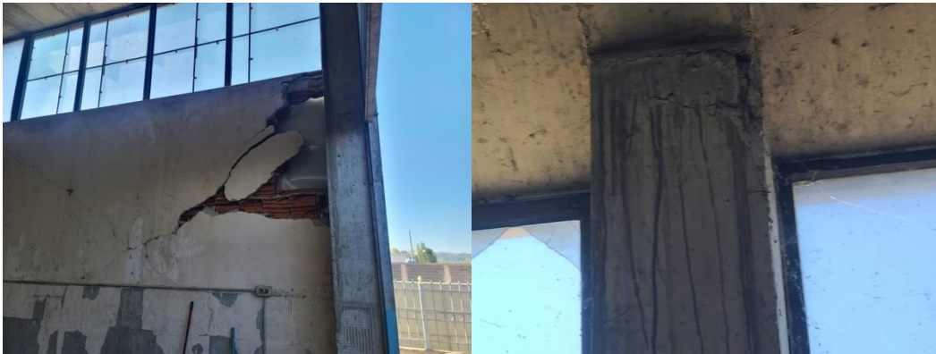
Figure 5. Wall and column damage on the first floor of the structure
