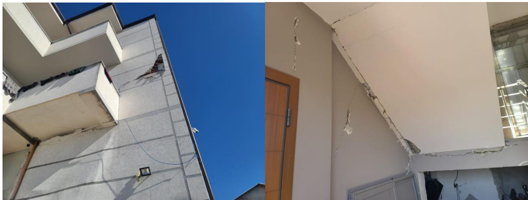
Figure 6. Damage on perimeteral walls of the façade
