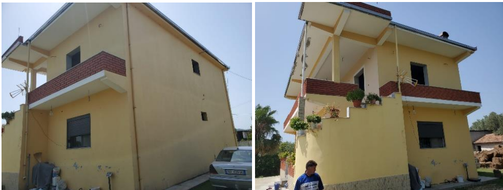
Figure 3. Damage patterns on CM building
