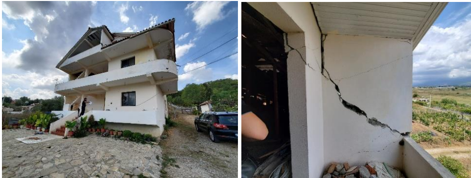
Figure 4. Damage patterns on RC building
