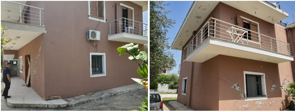
Figure 2. Damage patterns on URM building
